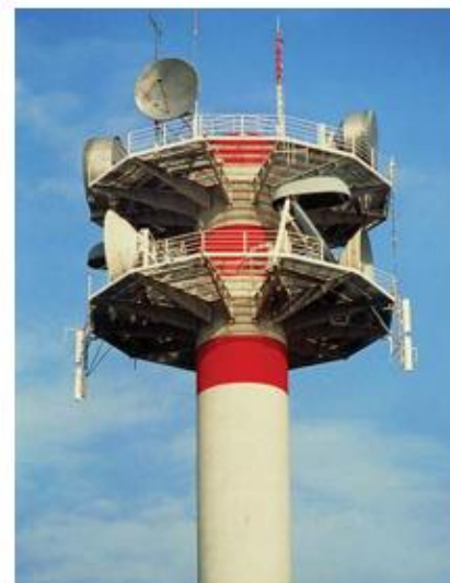
Figure 20.17 A microwave tower.
